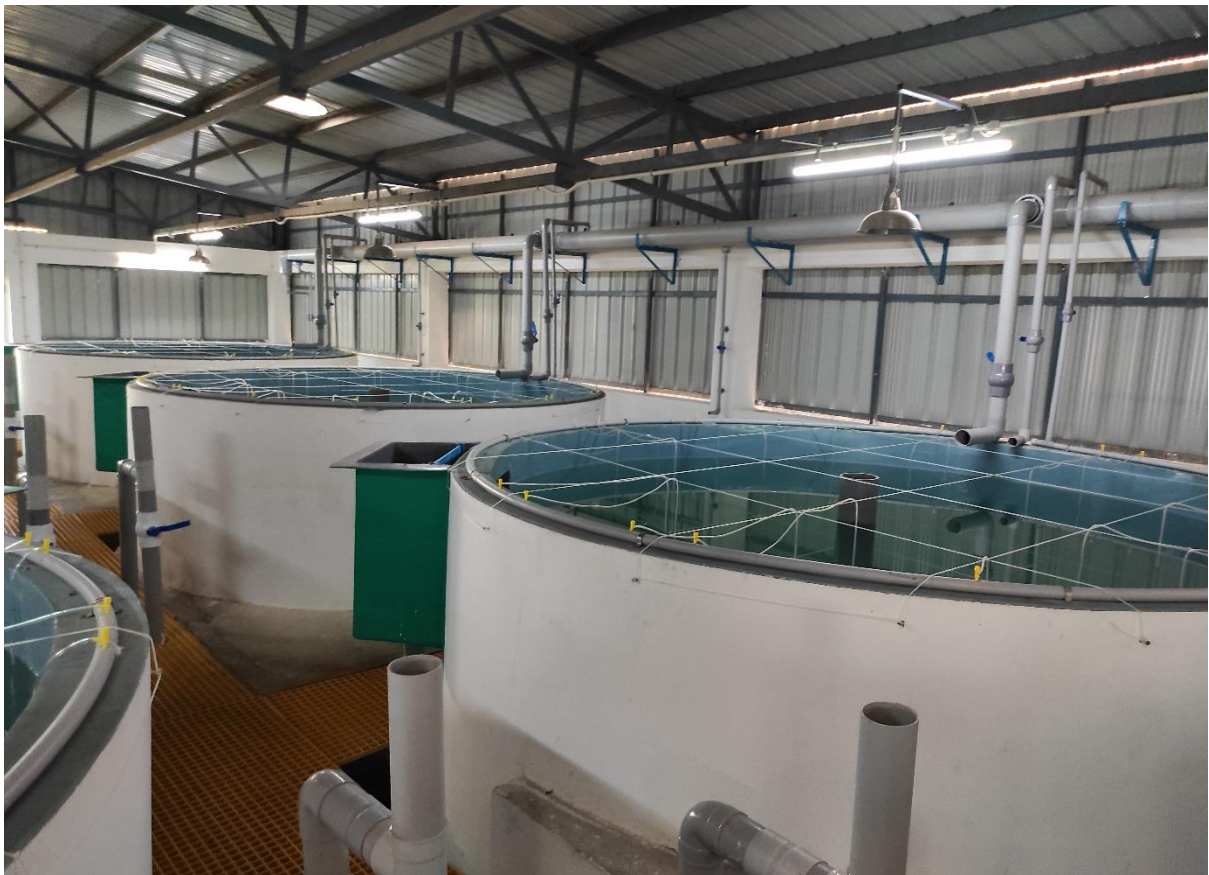
Inner view of RAS tanks
