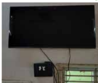
Installed SMART TV at Boys' Hostel
