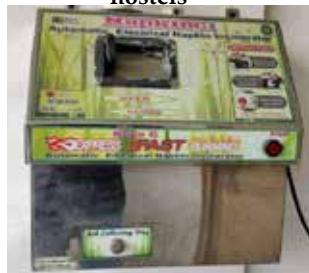
Re-installed Napkin incinerator
