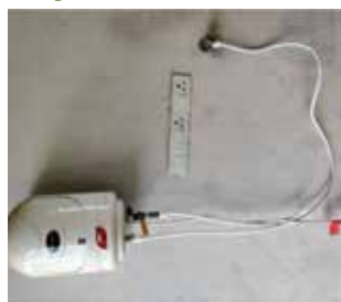
Installed Water Heater in hostels
